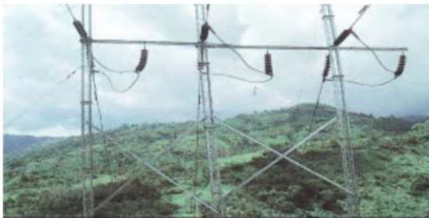
APEX - 69KV Transmission Line
