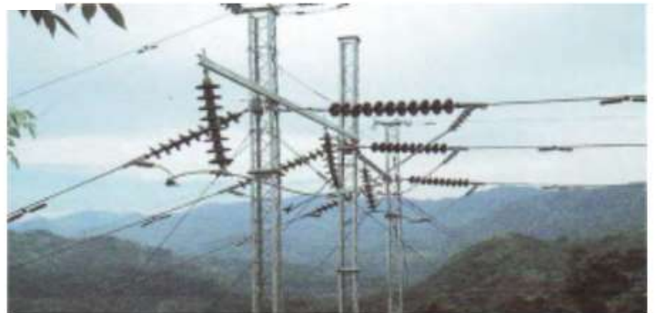
APEX - 138KV Transmission Line
